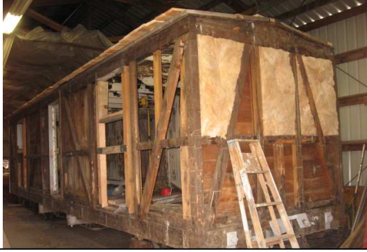
The bunk car did not originally have insulation. However, since we plan to use this car for crew accommodations, we felt a little modern insulation would be a welcome addition.
