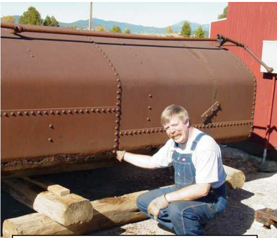
Mike Roberts pushing his hand through one of the tank car's rust holes that will be repaired in 2011
