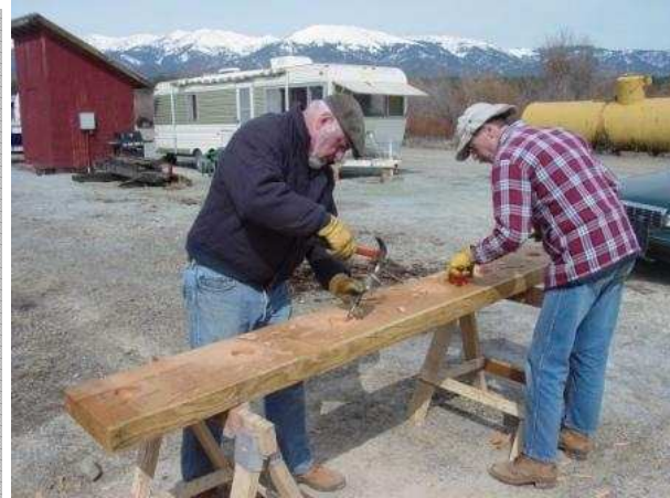
Ken Hittle and Kevin Rasmussen work on one of the last new deck boards to be installed.
