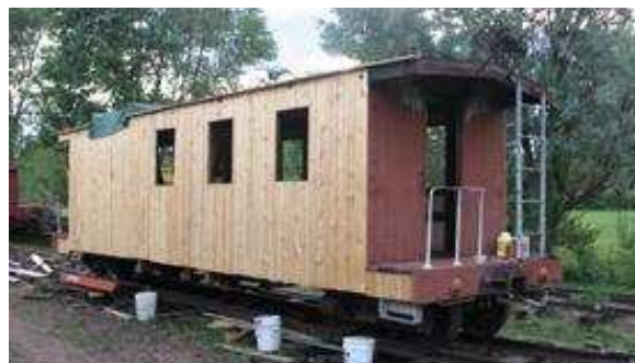
By July 11 th , our crew had all the new siding finished and were ready to begin building the new cupola. Jason Midyette photo
