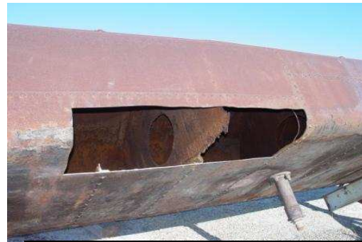
With the first rusted section of the tank removed, the badly rusted center tank baffle is visible – it will be replaced.
