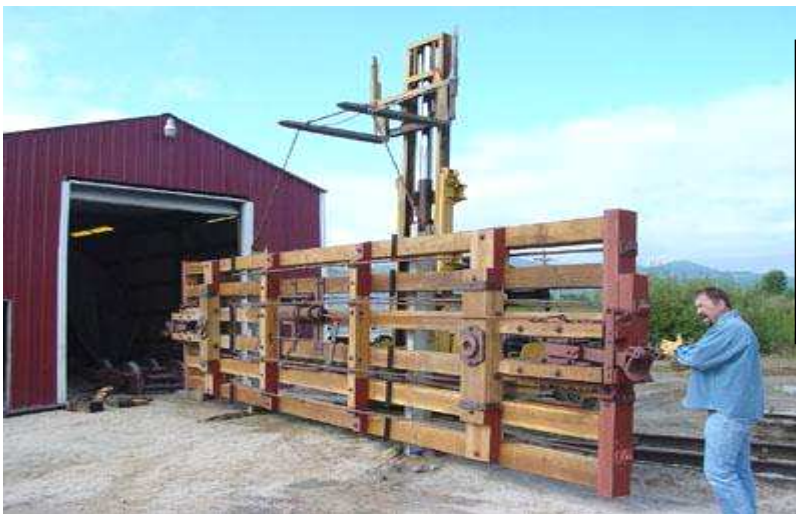
Jerry Huck helps to guide the forklift operator as the newly completed tank car frame is flipped right side up and placed on its trucks. Building the frame up side down allowed much easier installations of the car’s hardware.
